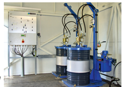
Pump station with barrel pumps and control unit
